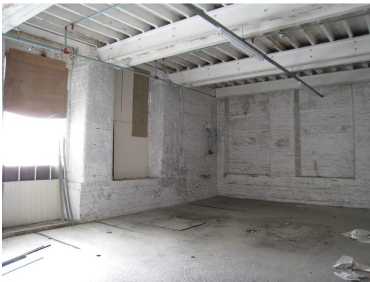
4.5 Quarini, C. State of four of the windows at Salts Mill on the first research visit in 2011, showing their appearance of gradually blocking up. Photo: C Quarini.
