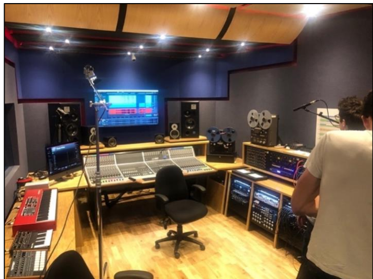
Fig. 37 RF07- Live control Room - Enid - Yes! (2021)
